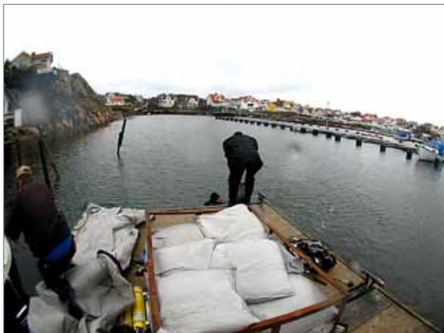
Figure 7. Sandbags used to stabilise the site. Photo Staffan von Arbin, Bohusläns museum.
